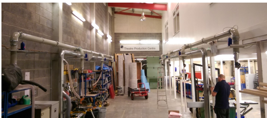
Installation showing the Inteliair™ controlled dampers
